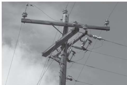
Deadly utility pole prior to retrofitting
